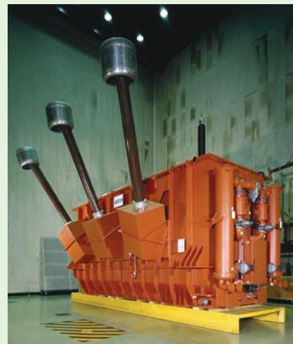
Figure 44.5 Step-up transformers at a power station
