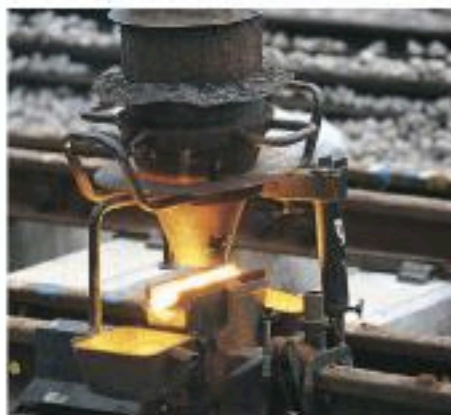
Figure 8.1 Rails are welded together using molten iron, produced by a reactivity series reaction between aluminium and iron(III) oxide.
