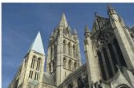
Figure 12.26 Weathering on the copper-covered spire of Truro cathedral.
