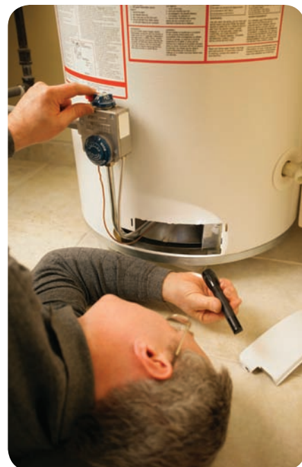
▲ Gas-fuelled water heaters and boilers should be checked regularly. Every year, hundreds of people are killed by carbon monoxide from faulty burners.
