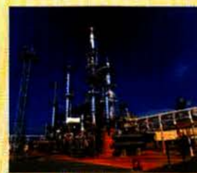
This is a plant for catalytic cracking. Such plants are often known as 'cat-cracker' plants.
